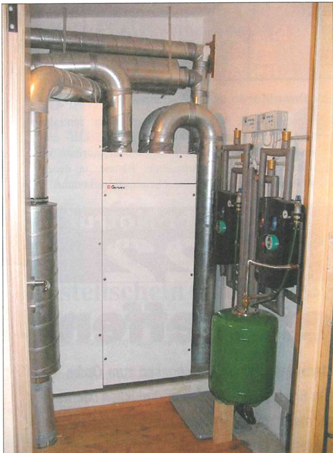
Haustechnikraum des Passivhauses Dipl.-Ing. Treichl, Schiefeling.
