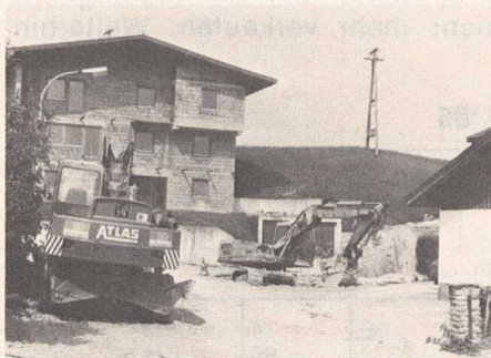
Kanalisation in Tafang
